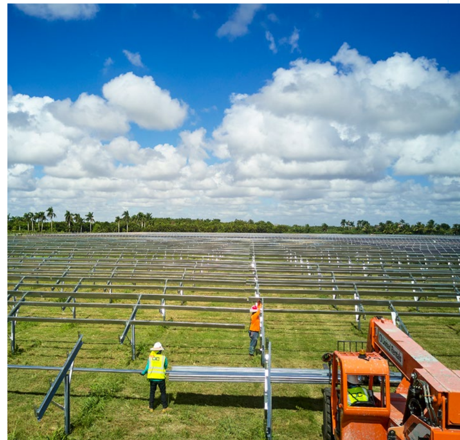
Crews construct what today is the FPL Miami-Dade Solar Center in Florida.
