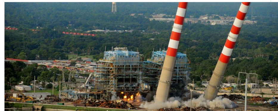
The distinct red and white stacks of FPL's Cape Canaveral Power Plant in Florida are demolished to make way for a more modern, efficient, less-carbon emitting facility to serve Florida customers.
