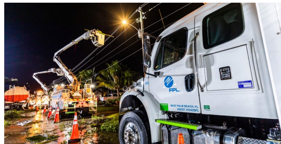
FPL crews work to restore power following a storm in West Palm Beach, Fla. Our emergency preparation efforts to strengthen the grid against storms and train for quick storm response increases reliability for our customers.
