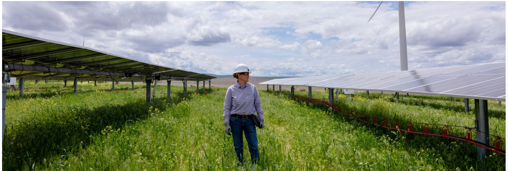
Employee Jana Lehn surveys solar panels at the Wheatridge Renewable Energy Facility in Lexington, Ore. The operation combines solar with wind and battery storage.
