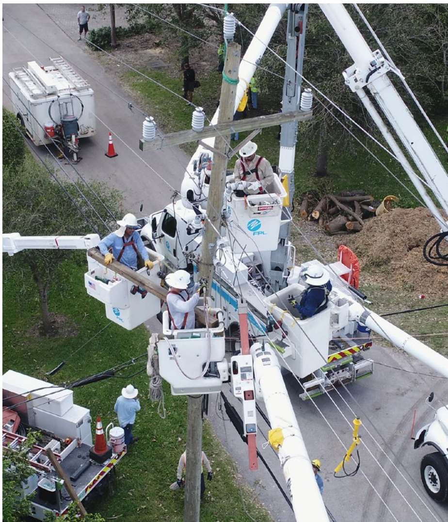
FPL line workers work to repair damaged power lines in South Miami-Dade County, Fla., after Hurricane Irma, one of the Atlantic's strongest and costliest hurricanes.
